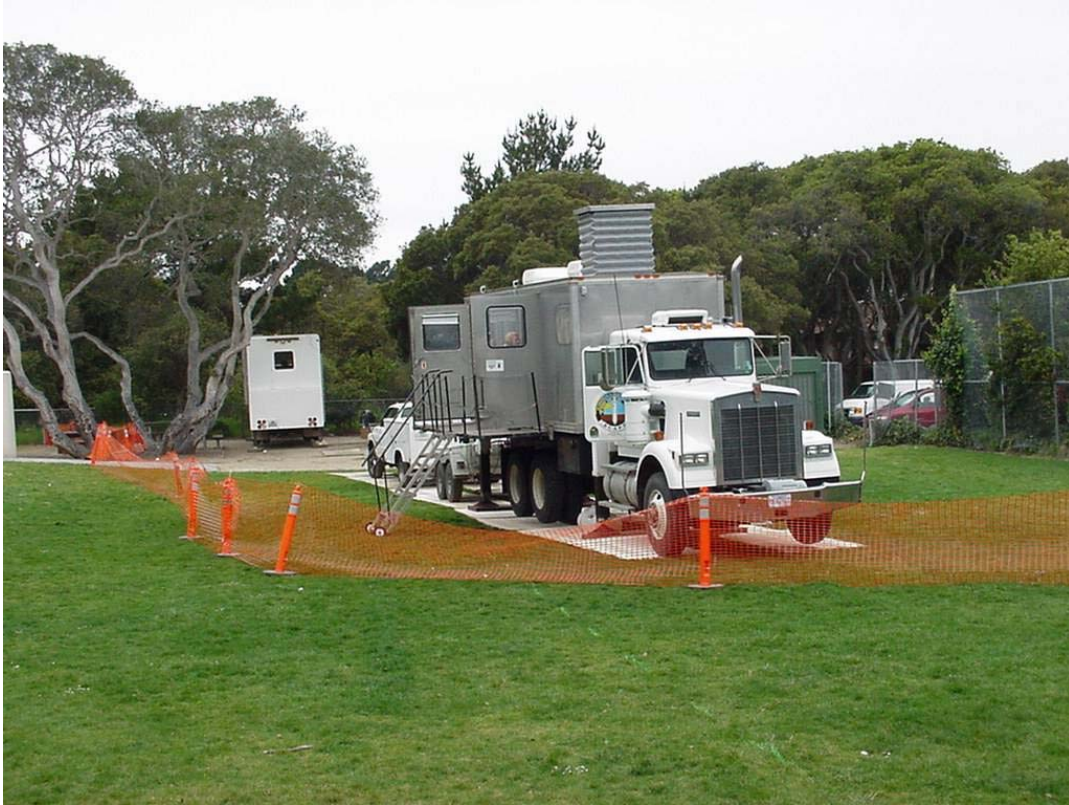
During the drilling, the area was fenced off from public access to the SCAPS truck.
