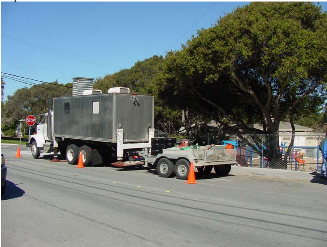
SCAPS unit is drilling in front of Casanova Oak Knoll Community Park.
